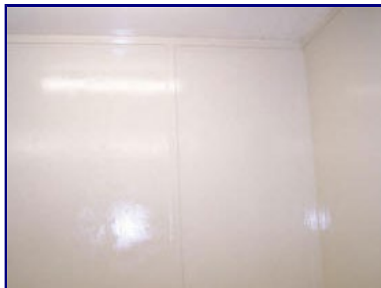
Epoxy.com Product #1 All Purpose Epoxy Coating on Plywood walls and Floors. Installation and Picture by: Suwannee River Rendezvous Resort & Campground
